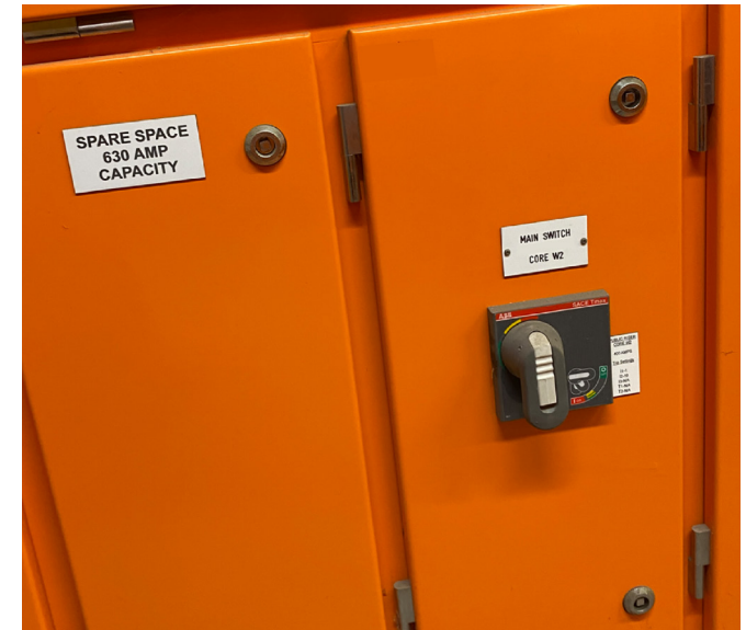
This 630Amp MSB spare was utilised for a 350kW battery.
